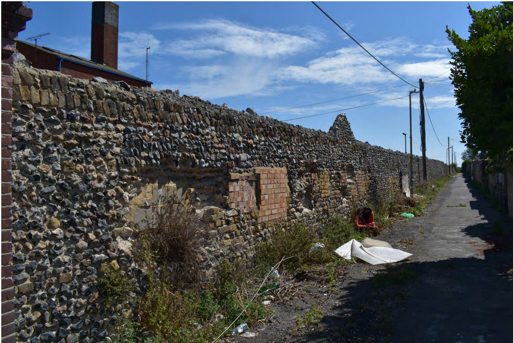
Plate 18: Southern side of the Bungaroosh wall from the public footpath (facing east)
